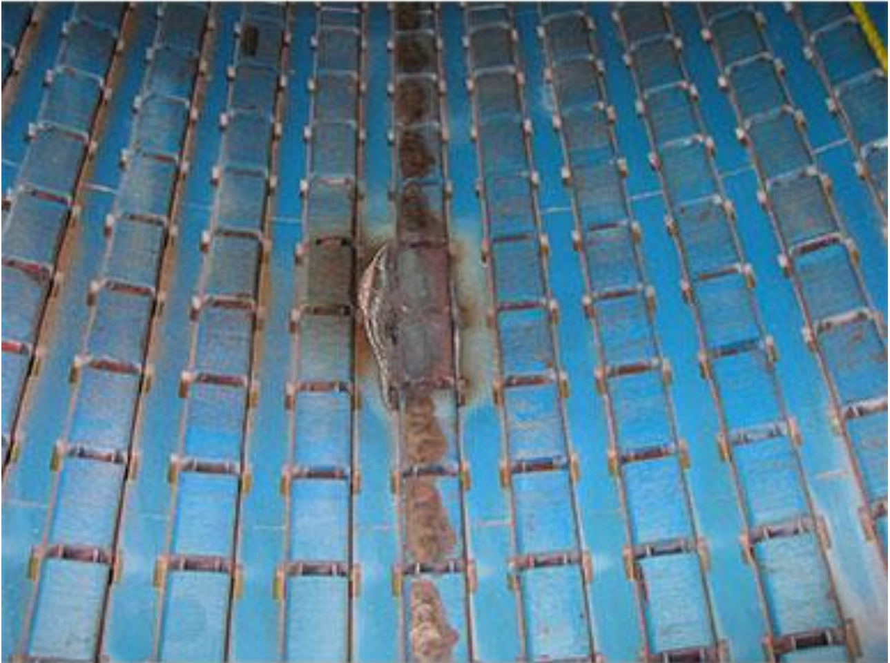
Figure 3 – Burnout of TG stator winding, which led to damage to the core package [6]
