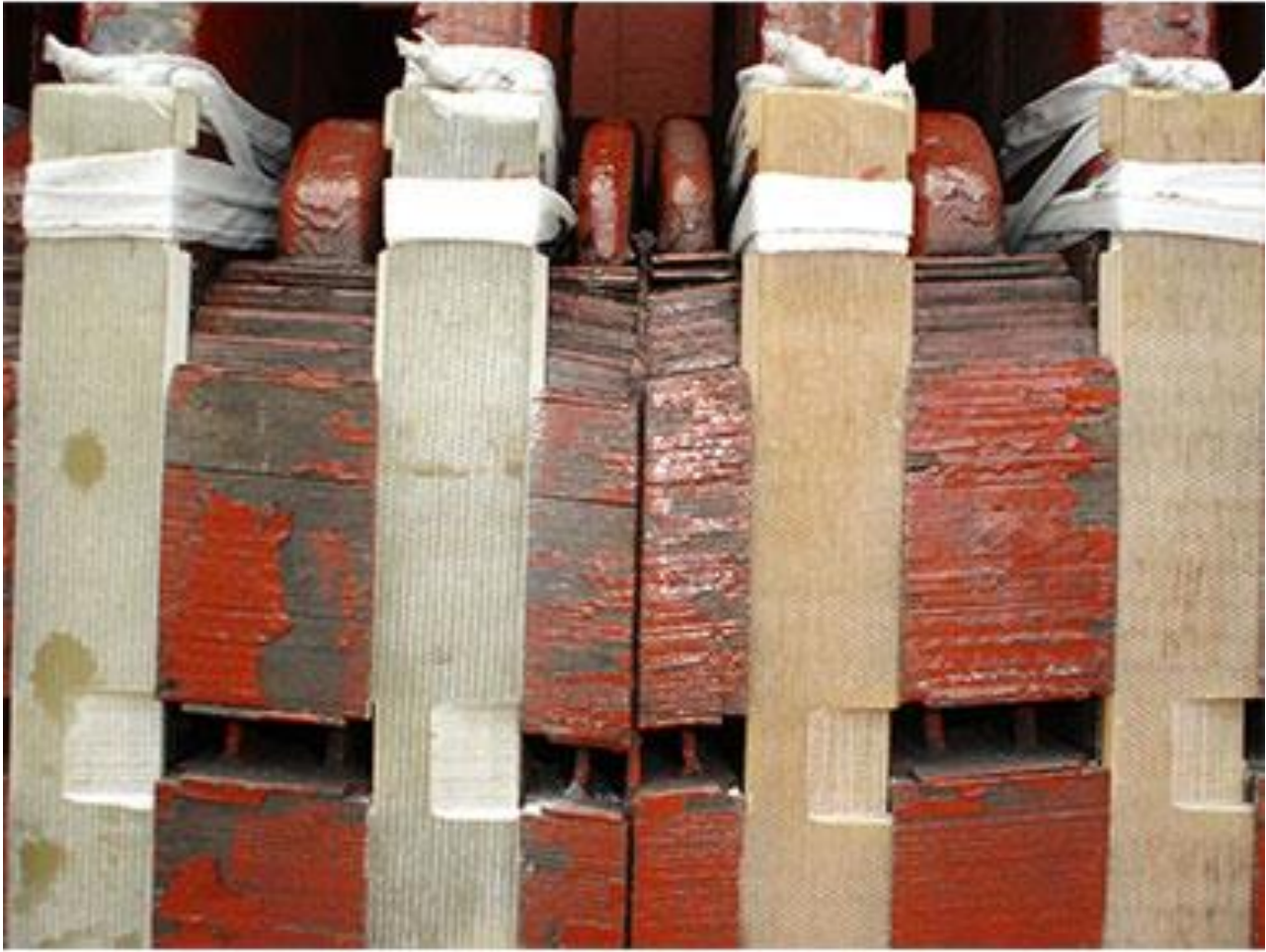
Figure 4 – The stator core end damage [6]
