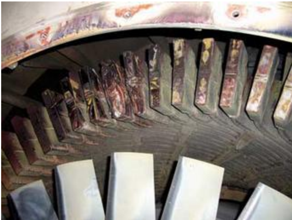
Figure 2 – Damage of the front part Toshiba TG stator winding insulation with a capacity of 124 MVA [4]
